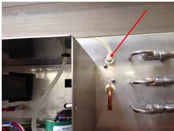
Figure 3.4 - Flowmeter outlet tube
