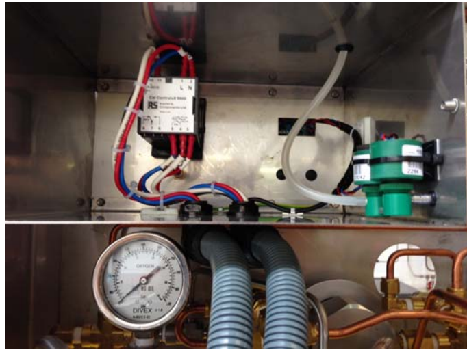
Figure 3.7 - Modified upper electrical enclosure
