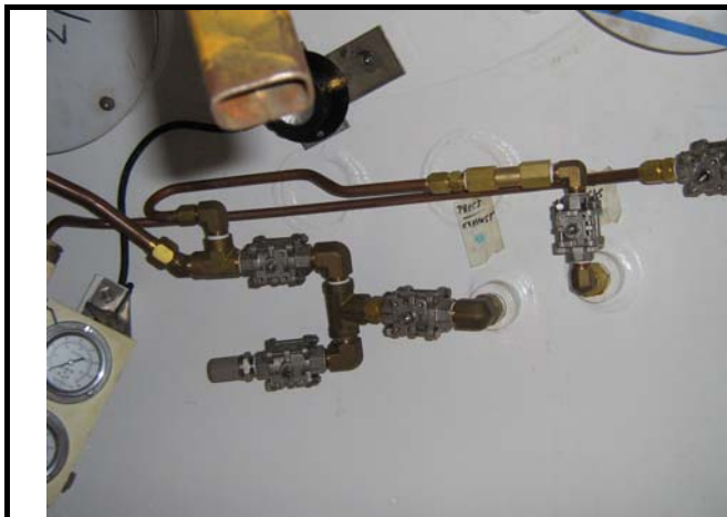
High Pressure lines (3,000psi) and Low Pressure lines (1,000psi) are located in the same area.
